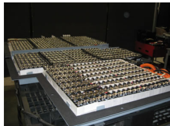
Coda Sedan 34kWh Battery System
